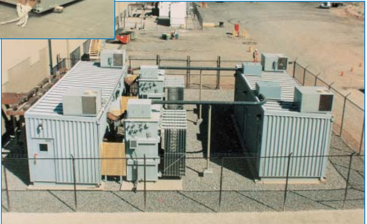
40,000 amp DC, 220 VDC 12 pulse electro-winning installation with oil-filled transformers and harmonic filter
