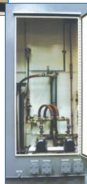
Water to water heat exchanger
