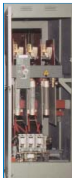
High voltage fused disconnect switch
