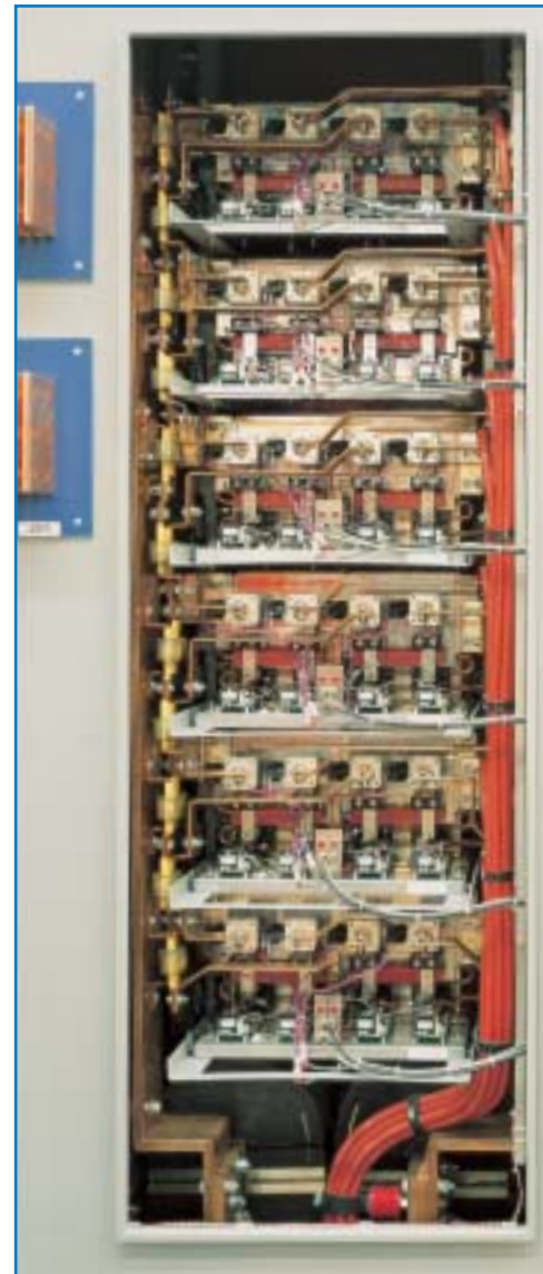
The above is a section of a 36,000 amp chopper system used on a graphite furnace application.
