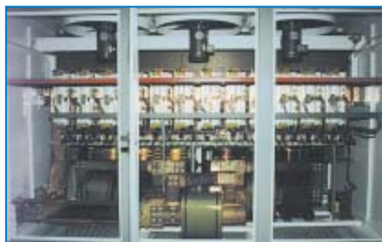
16,500 amp air-cooled thyristor rectifier
